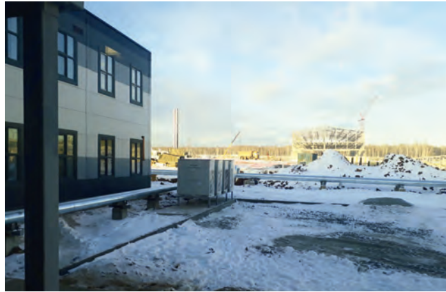
Tominsky Mining and Refining Plant, Chelyabinsk region Hitachi VRF Set Free
