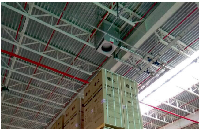
Warehousing facilities of the LG company, Ruza, Moscow region Decentralised ventilation system Hoval
