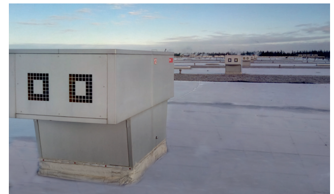
Finished products warehouses of the KDV confectionery factory, Voronezh region Decentralised ventilation system Hoval
