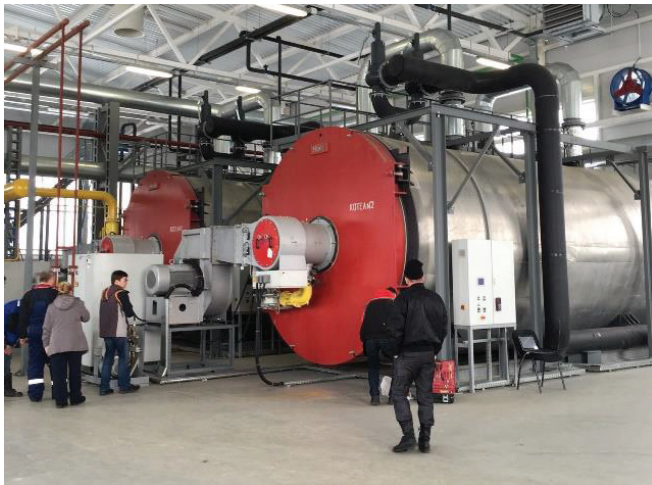
Boiler house, Residential complex»Domodedovo», Moscow region Autonomous gas boiler room with a thermal capacity of 36.12 Gcal/h. Equipment supply
