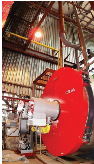
North Domodedovo Hoval Boiler equipment Equipment supply
